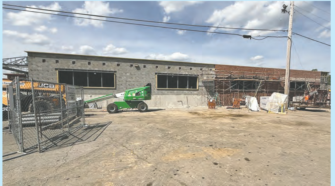
Jefferson Elementary continues its renovation and expansion project to modernize the school's facilities and improve accessibility for all students. (See story on page 3)
